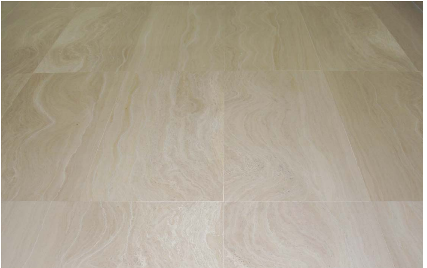
Italian Marbre pavement in flats, ground floor, first floor and second floor
